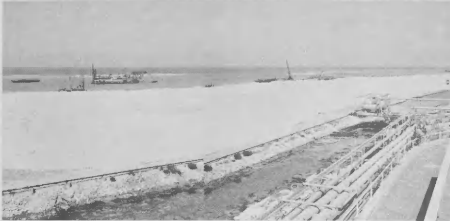
Dredge "Georgia", working for Netherlands Harbour Works, began dredging and land reclamation work on April 2, 1969.
